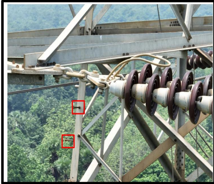
Rusting on Footstep bolts
