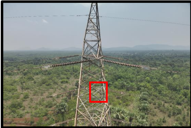
Bird Guard is Missing
