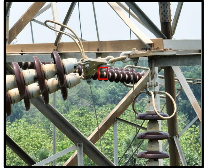
Tie pin is missing
